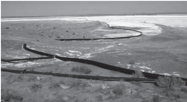
Figure 2a On-grade Installation of PE Pipe in an Industrial Application. Note "snaking" along right of way.
