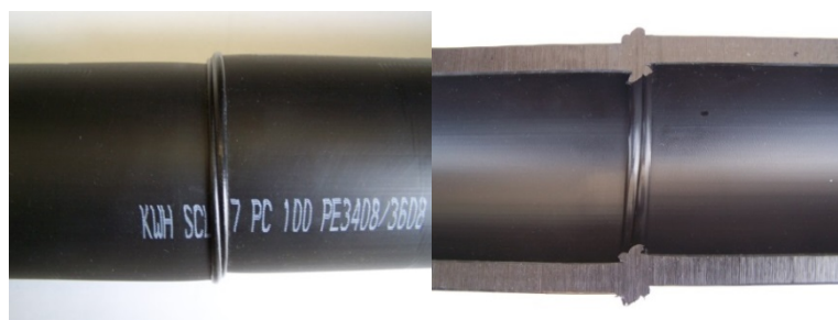
Figure 7 - Pipe misalignment (high-low misalignment)
