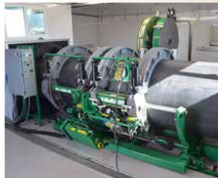
Machine operator and fusion joints are protected from the elements inside the shelter.
