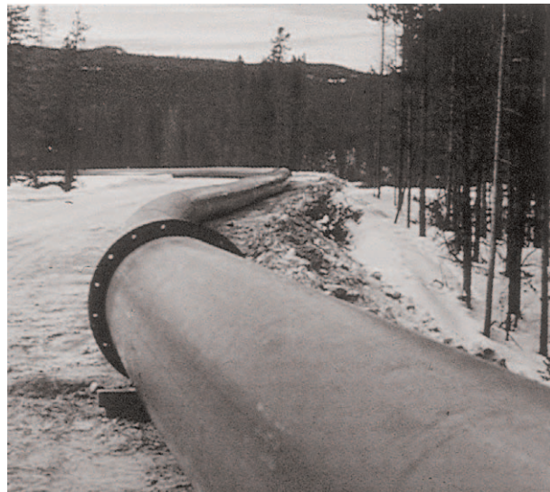
In this mine tailings applications, 36 inch series 60 SCLAIRPIPE is installed at grade on a prepared right of way. The pipe routing incorporates a number of gentle bends to accommodate thermal expansion and contraction forces, minimizing the overall stresses on the pipe.
