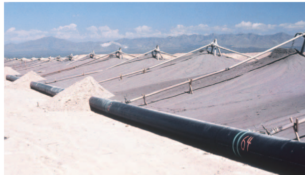
SCLAIRPIPE used in a tailing applications at a molybdenum mine in Arizona. Inclusion of 2% finely dispersed carbon black ensures that the pipe is resistant to ultraviolet light degradation enabling it to be installed at grade. Anchoring of the pipeline is achieved simply by dumping a load of tails on the pipe at regular intervals.
