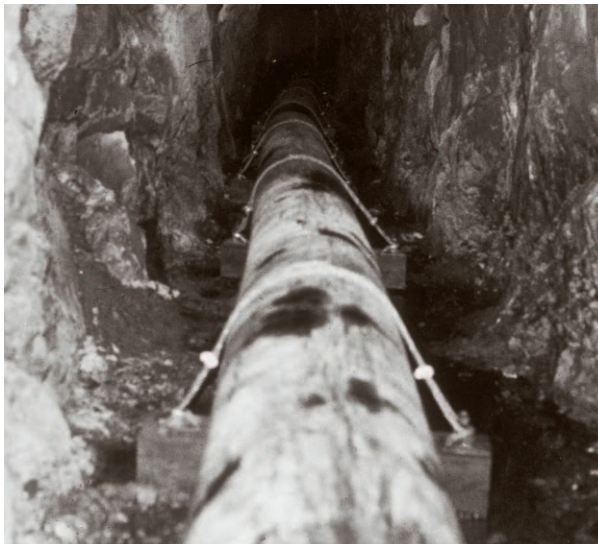
At Kirkland Lake in Northern Ontario, a gravity sanitary sewer of 18 inch SCLAIRPIPE is installed in a rock tunnel. Pipe is laid above ground, tied down to wooden sleepers and secured with rock anchors.
