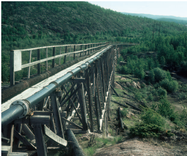
Installation of this 8 inch series 125 SCLAIRPIPE tailings line called for it to be supported on a trestle to maintain grade. Note the guides located at regular intervals to hold the pipe on the trestle during thermal expansion and contraction situations.
