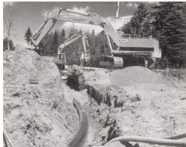
SCLAIRPIPE was the material of choice for a 20 mile brine line running from a potash mine in Sussex, N.B. to the Bay of Fundy. The line was installed without surge protection devices although it included sections operating in excess of 200 psig.
