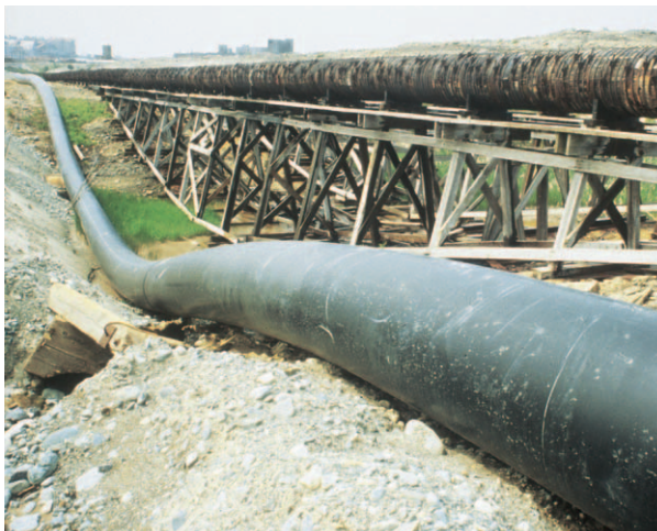
28 inch series 60 SCLAIRPIPE was used to replace a woodstave line at a mine site in Noranda, Quebec. This 10,000 foot water supply line had a design pressure of 50 psig and was installed in 1978.
