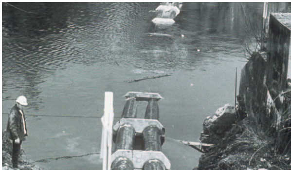
Installation of 24 inch SCLAIRPIPE for a twin sewage siphon line in Victoria, B.C. The pipe is completely resistant to seawater and its smooth surface discourages the adherence of algae and other marine growths.
